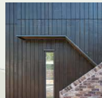
Black stained weatherboard
