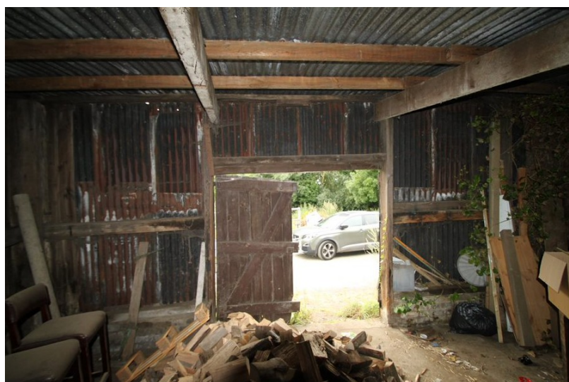
Fig. 14. The entrance to the shed looking south (image provided by Chris Saunders).
