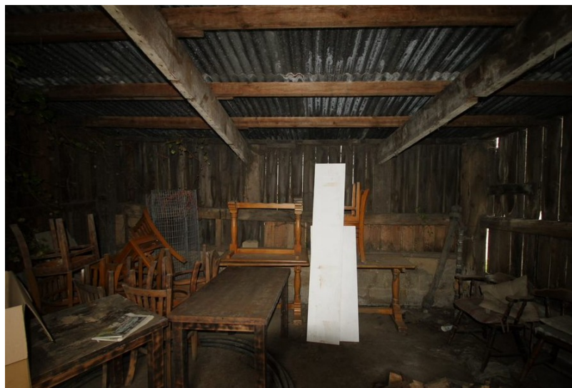
Fig. 13. The inside of the shed with block-work plinth (image provided by Chris Saunders).
