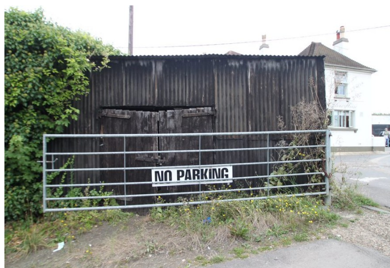
Fig.11. The south facing entrance to the shed (image provided by Chris Saunders).
