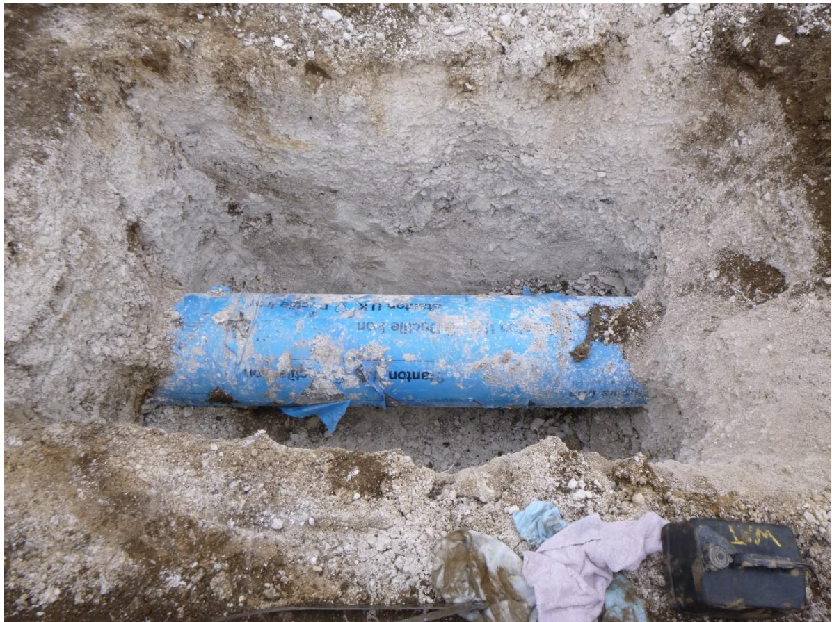
FIGURE A1.3 – EXCAVATION AT INSPECTION SITE, STANGUARD WRAPPING IN GOOD CONDITION
