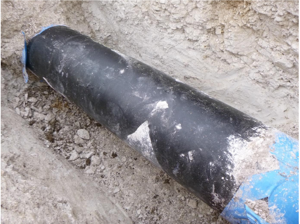
FIGURE A1.4 – PIPE SURFACE BENEATH STANGUARD, GOOD CONDITION
