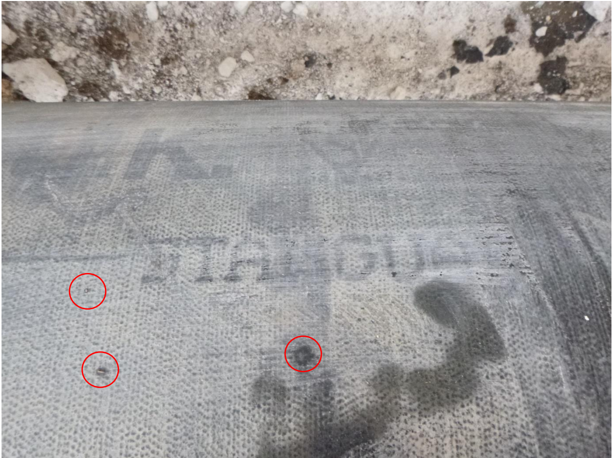
FIGURE A1.6 – CLOSE UP OF PIPE SURFACE, SUPERFICIAL EXTERNAL DEFECTS NOTED
